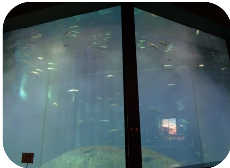
Cloudy acrylic panels and deterioration of glued parts
