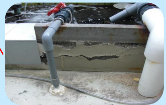
Deterioration of concrete (of the water tank)
