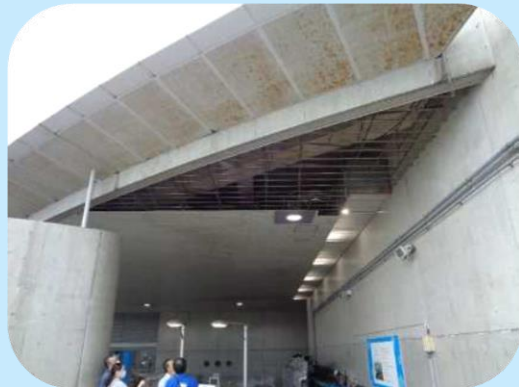
Corrosion of the ceiling bed *It has been repaired as of March 2023.
