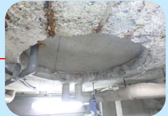
Corrosion of reinforcing steel and deterioration of concrete
