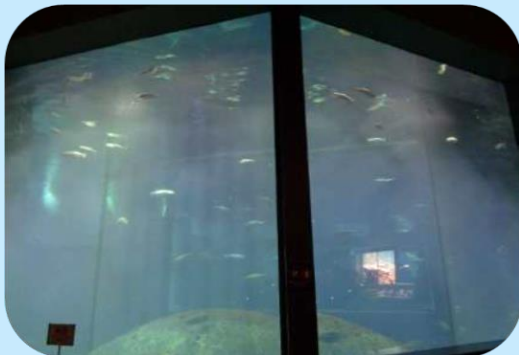
Cloudy acrylic and deterioration of glued parts
