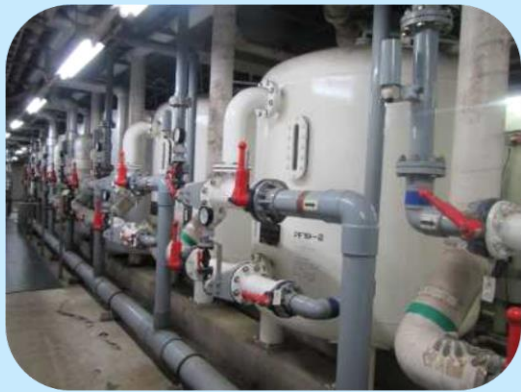
Filtration tanks are placed close to each other.
